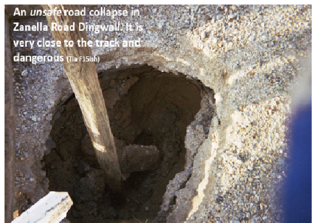
Figure 13: An example of unsafe infrastructure source: 'week with a camera' participant
