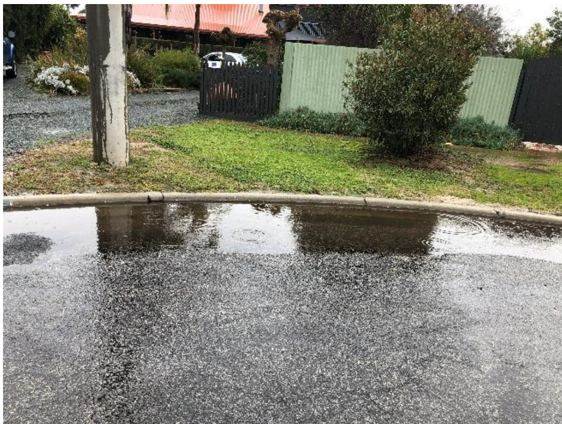
Stormwater ponding during light rain at Fehring Court, Cohuna
