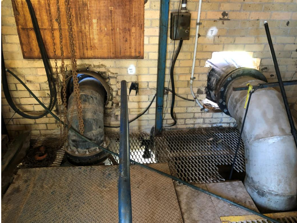
Pump outlets at Wyndham Street, Kerang
