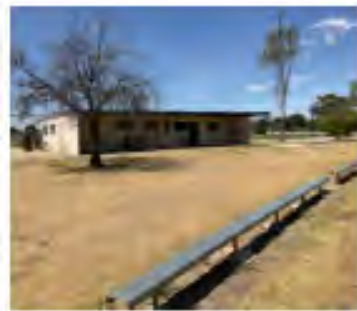
Condemned change rooms
