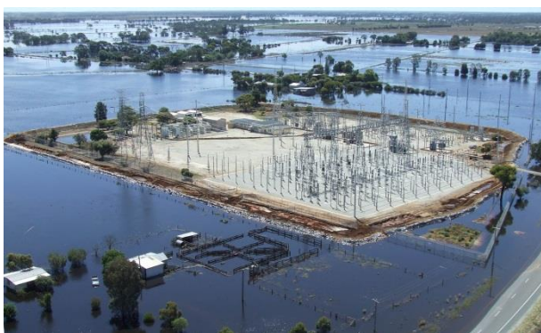
Photo above: Kerang Power Sub-station, Jan 2011 (photo courtesy Gannawarra Shire Council)
