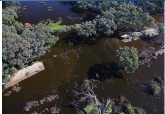
Above: Breach in the Lower Loddon Levee, Jan 2011 Flood (photo courtesy North Central CMA)
