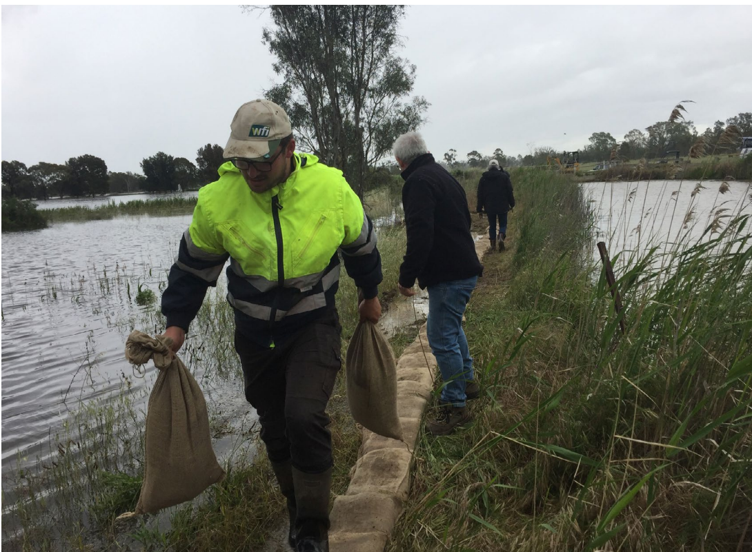
Left: Community members working to sandbag containment lines preventing the floodwaters (left) from entering the Goulburn-Murray Water channel (right) which would have impacted a greater number of homes, properties, private and public infrastructure, and the nearby township of Murrabit.
